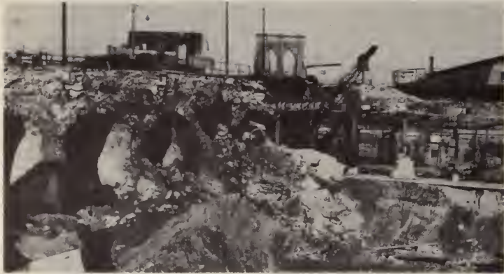
The old brick arches between Prospect Street and Sand Street are removed preparatory to changing the direction of the approach to come to grade at Adams Street instead of Fulton Street, the former approach street.
